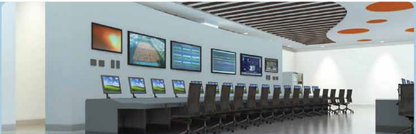
The artistic impression of the control room when the power plant is operational
