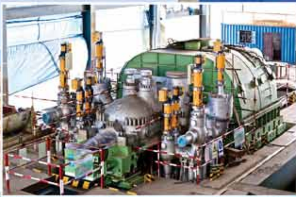
The 300 MW thermal power plant turbine with the casing
