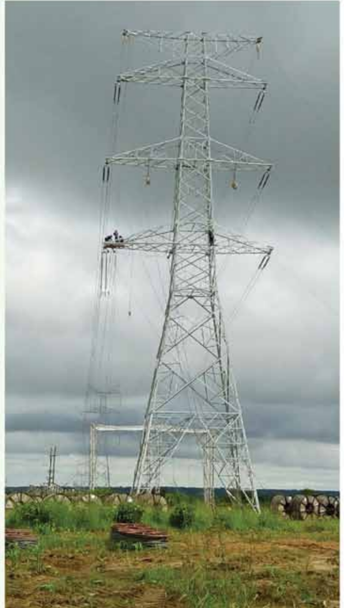
The newly constructed 330kv power line from Maamba to Izuma Conductor pulling works
