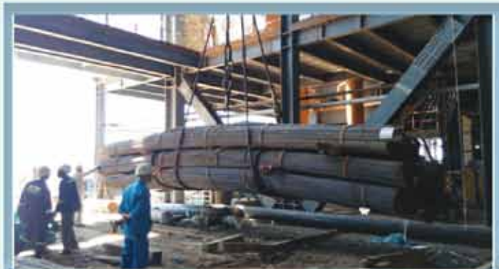
The tests ensure that the system is able to withstand high pressure and super heat temperatures.
