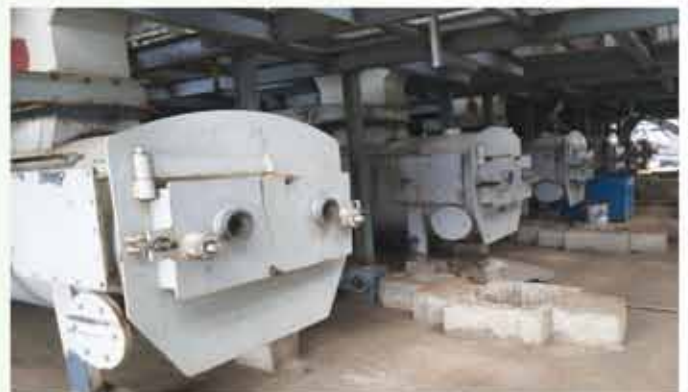
Unit-1 coal feeders
