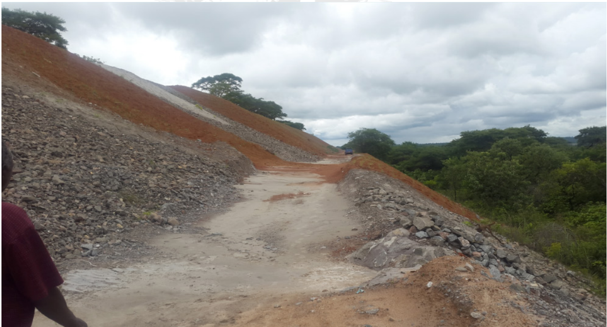
Photo 1: Improving access to safe drinking water in Sinda District of Zambia Rehabilitated Gullies at TD 10- Mufulira
